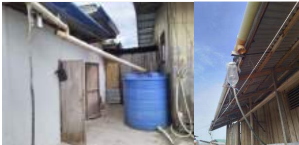
Figure 5. Existing rainwater harvesting systems, Sitangkai Source: ESIA Study
